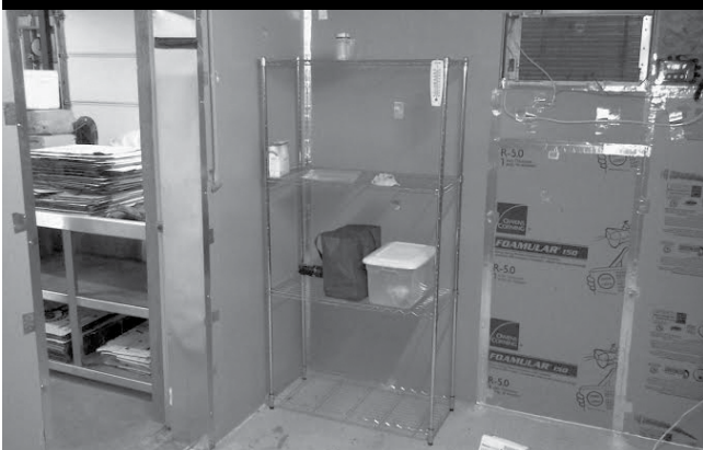
The walk-in cooler at Blue Gate Farm
