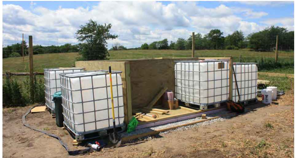
Construction of the compost heat extraction system. When completed, the unit will be insulated and closed, only opened to "fluff" or refresh compost.
